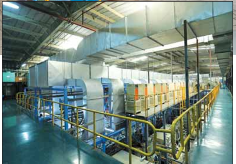
Auxiliary Equipment, Plating line
