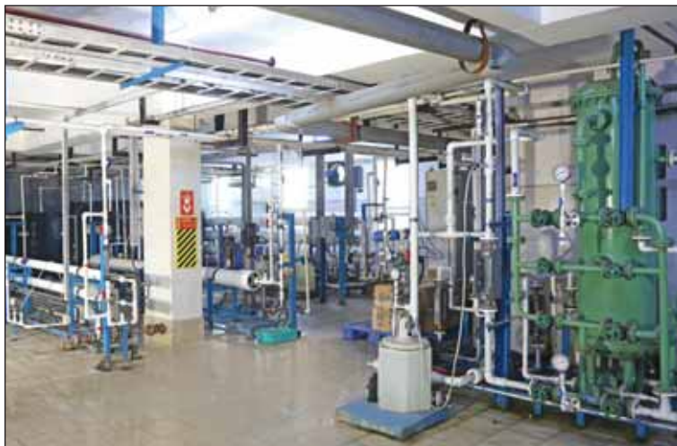
Effluent treatment plant with water recycling system
