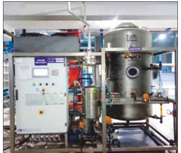
Vacuum evaporator for Chrome recovery
