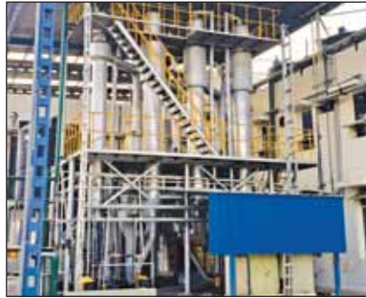
Zero discharge System
